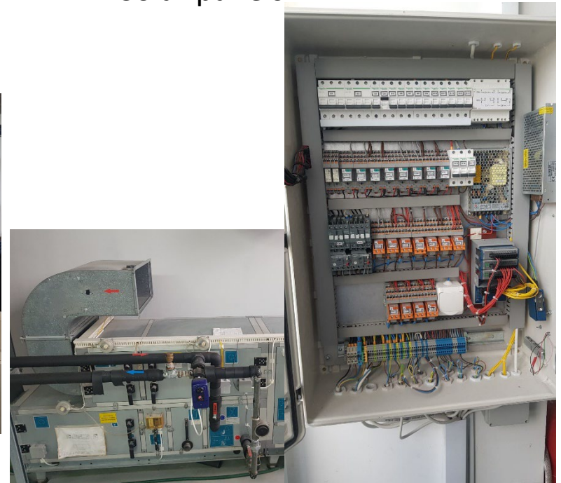
Automated heat pump
